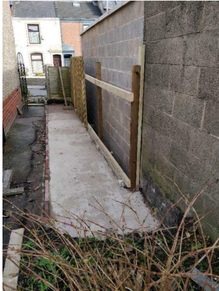
Figure 2: Extent of Unauthorised Hardstanding Installed by the Applicant
